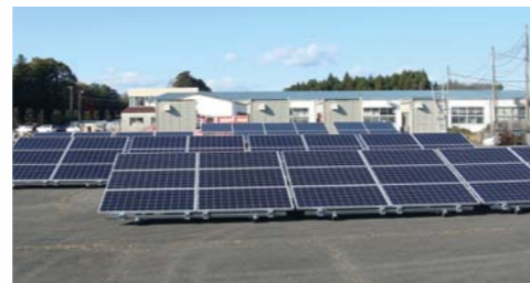
Test combining PV panels and solar inverters
